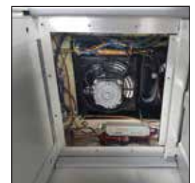
A5. Condenser compartment
